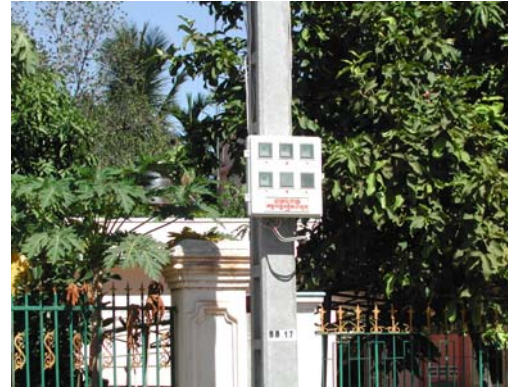
Metering System after Improvement
