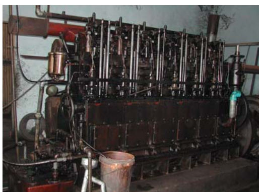
Generator Set before Improvement
