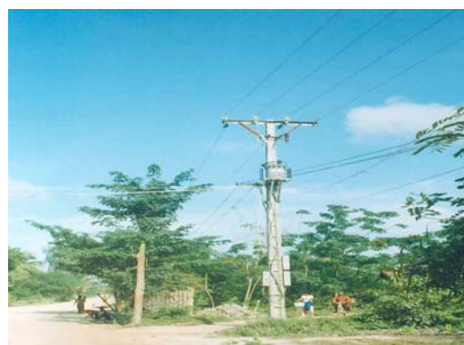
Medium and Low Voltage System after Improvement
