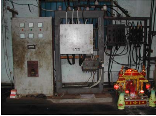
Control Panel before Improvement
