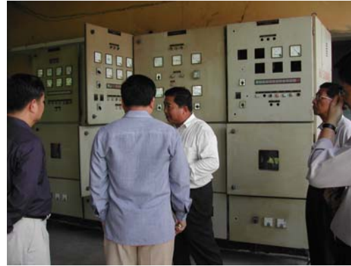
Control Panel after Improvement
