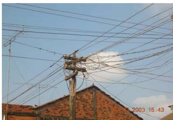
Low Voltage System before Improvement
