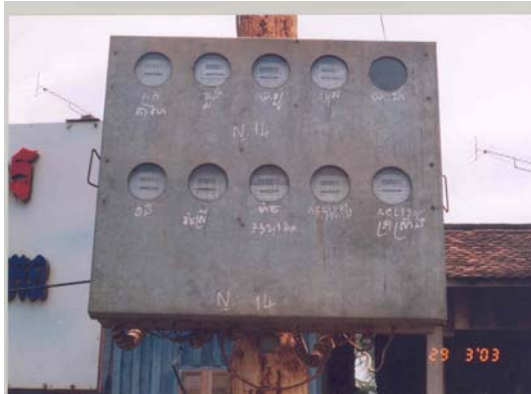
Metering System before Improvement
