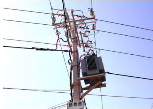
Medium and Low Voltage System after Improvement
