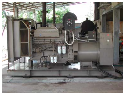
Generator Set after Improvement
