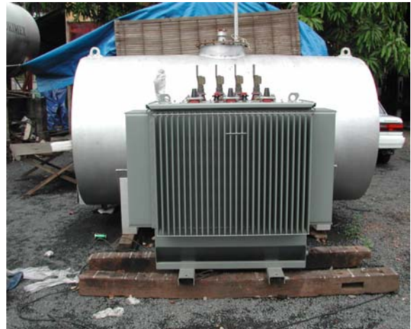
Electricity Equipment for Improvement
