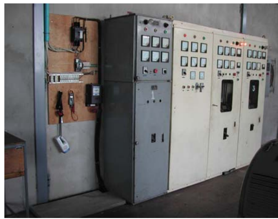
Control Panel after Improvement
