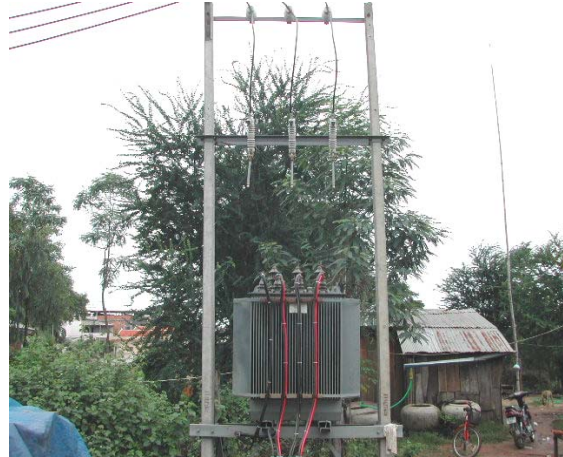
Transformer after Improvement
