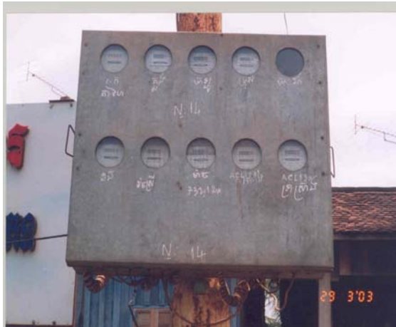
Metering System before Improvement
