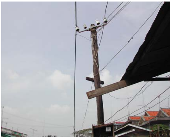
Low Voltage System before Improvement
