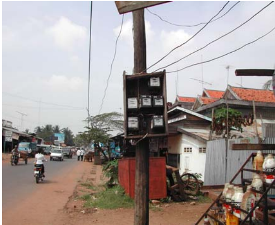
Low Voltage System before Improvement
