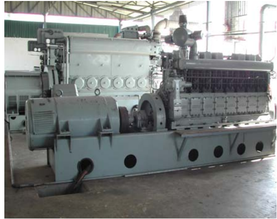
Generator Set after Improvement
