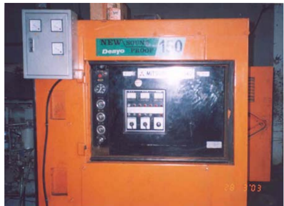
Generator Set after Improvement
