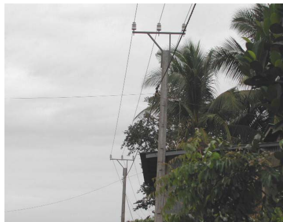
Medium Voltage System after Improvement
