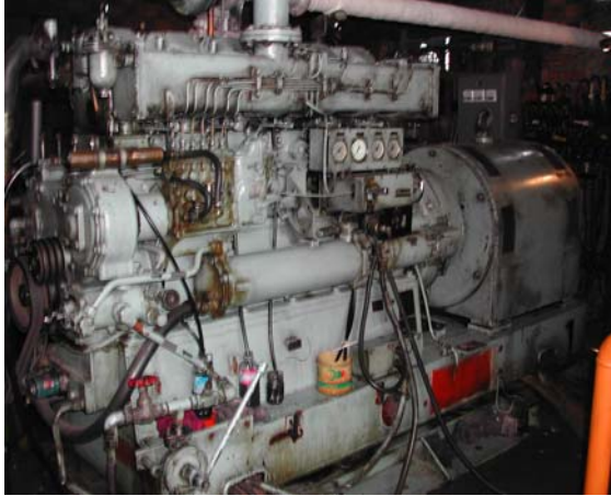
Generator Set before Improvement
